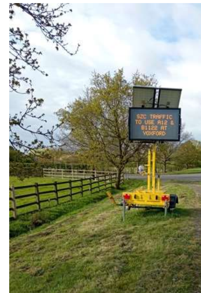
Site 2: Darsham VMS Sign installed on A12, near Darsham with The Street.
